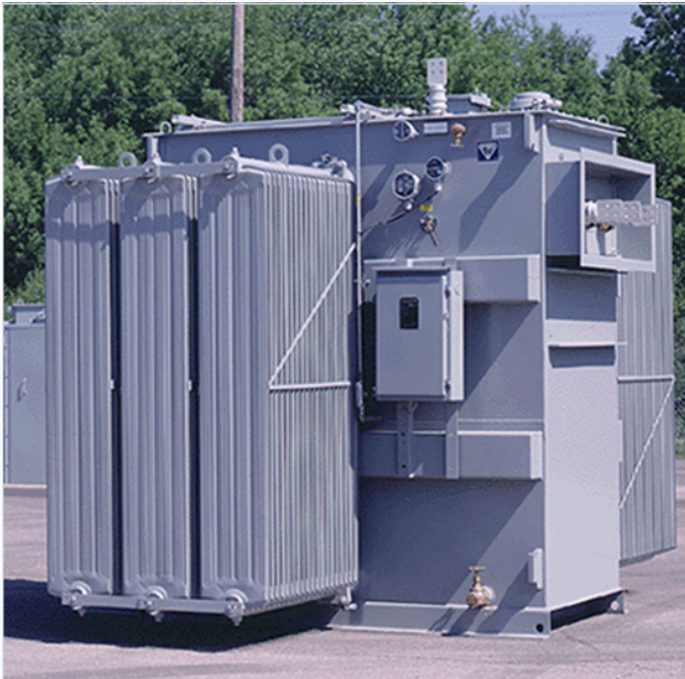
Oil-filled substation transformer 14
