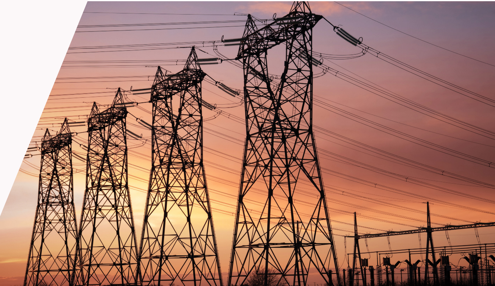
Section of transmission lines
