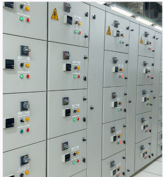
Example of an MCC
