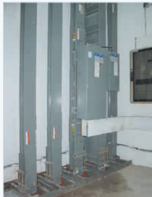
Example of a vertical busway riser 10
